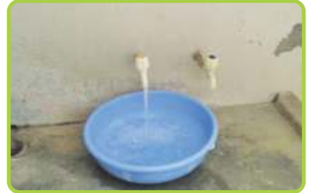
Drinking Water Tap connection- Tappar (Home of Mr. Mayursinh Jadeja)
